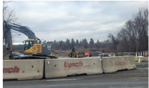
NEW HOSPITAL: Encompass Health has started clearing land for construction of a 50-bed inpatient rehabilitation hospital at 2109 Hartford Ave. in Johnston. (Sun Rise photo by Rory Schuler)
